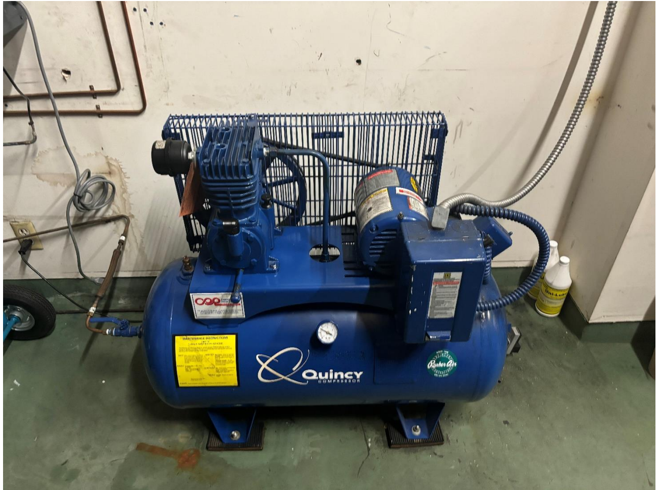
Air Compressor in Mechanical Room on 2 nd Floor
