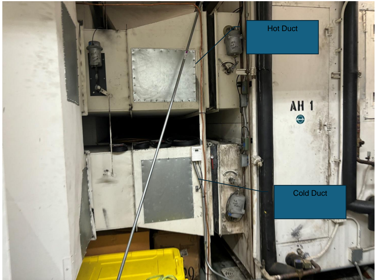
Air Handler Unit in the Mechanical Room on 2 nd floor showing double duct system.
