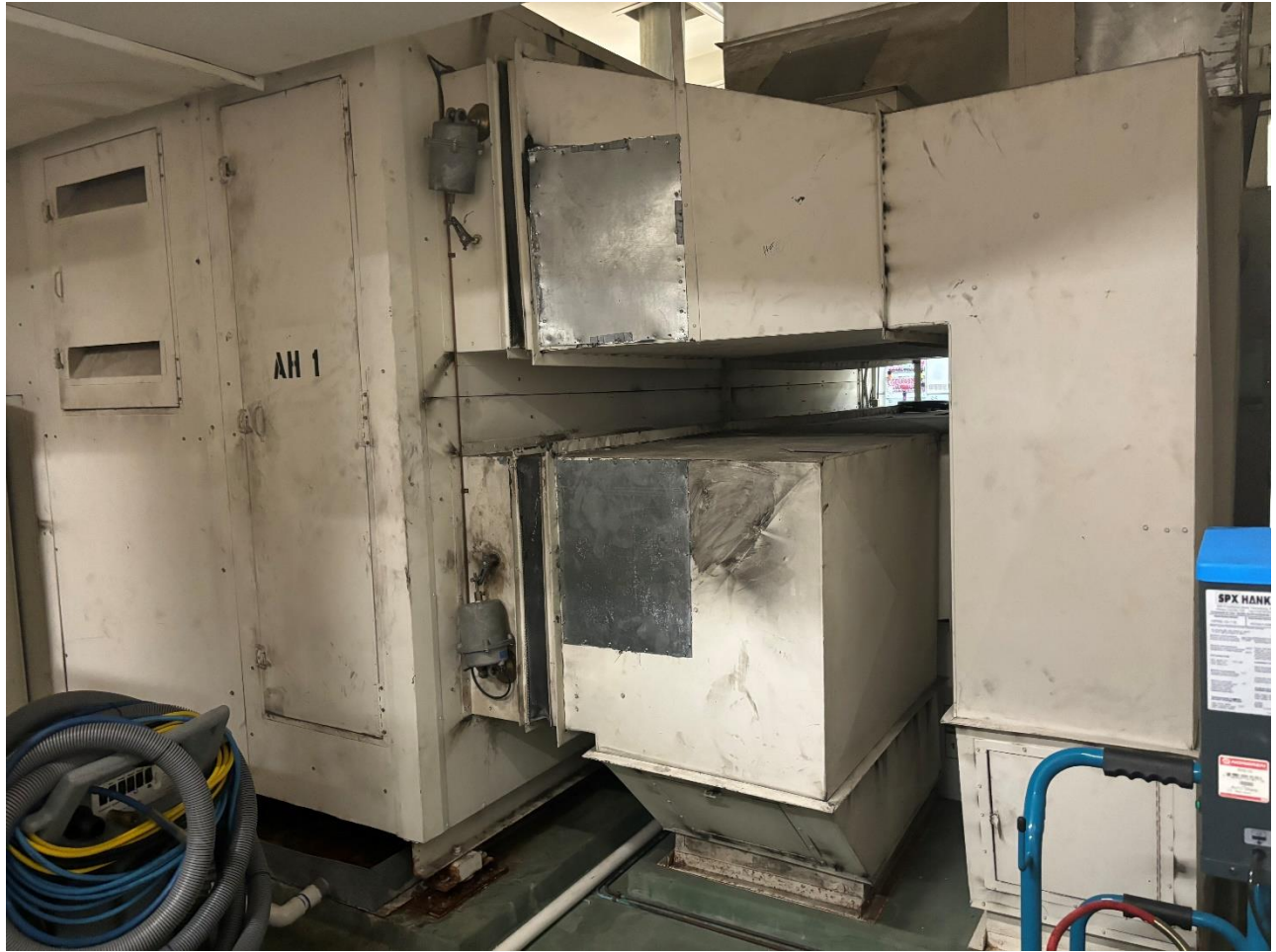
Air Handler Unit in the Mechanical Room on 2 nd floor
