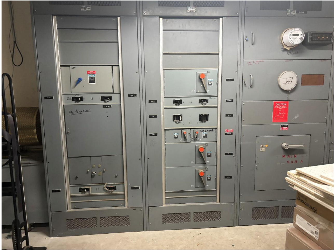
Electrical Room Panels on 2 nd floor
