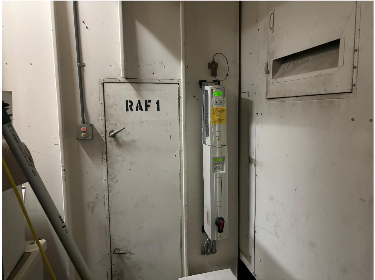
Return Air Fan in the Mechanical Room on 2 nd floor
